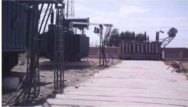
A view of the yard of Qila Safiullah Grid Station
